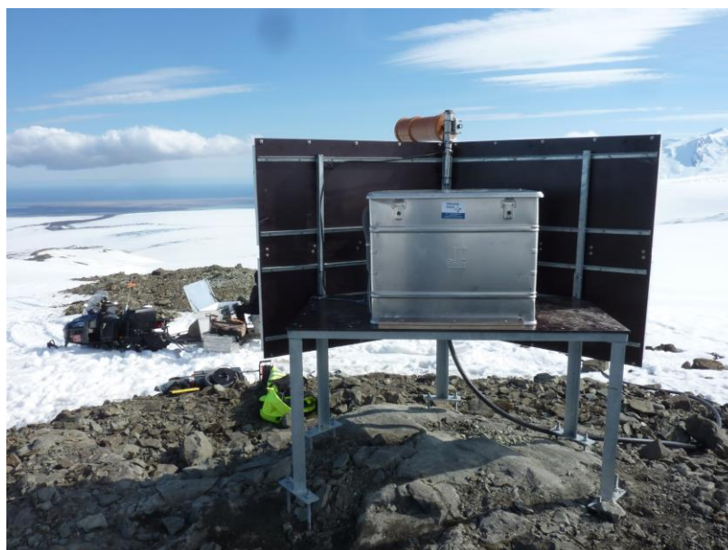
Figure 3. Photo of the setup at station ksk. In the foreground are the solar panels mounted on the frame carrying the batteries and electronic equipment. The frame is raised to protect the equipment from surface melt water. A brown plastic cylinder covers
